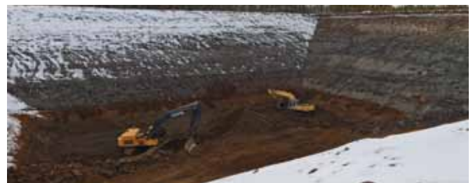
Late-stage construction of bulk sample pit in March 2011. (Photo courtesy of Dan Christal)
